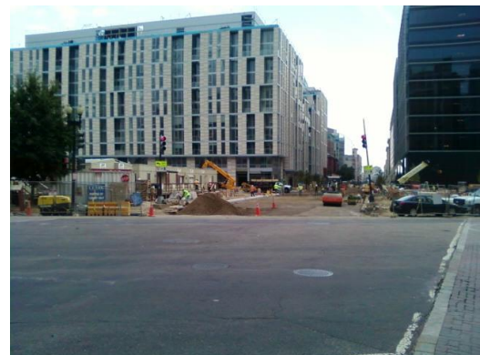
Crews prepare 10th Street to be re-opened between H Street & NY Avenue, NW.
